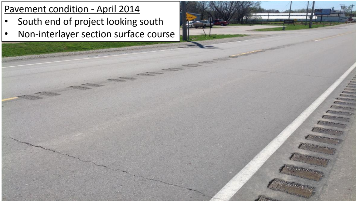
Figure 27. Photo of reflective cracks in non-interlayer overlay on US 169 in April 2014
